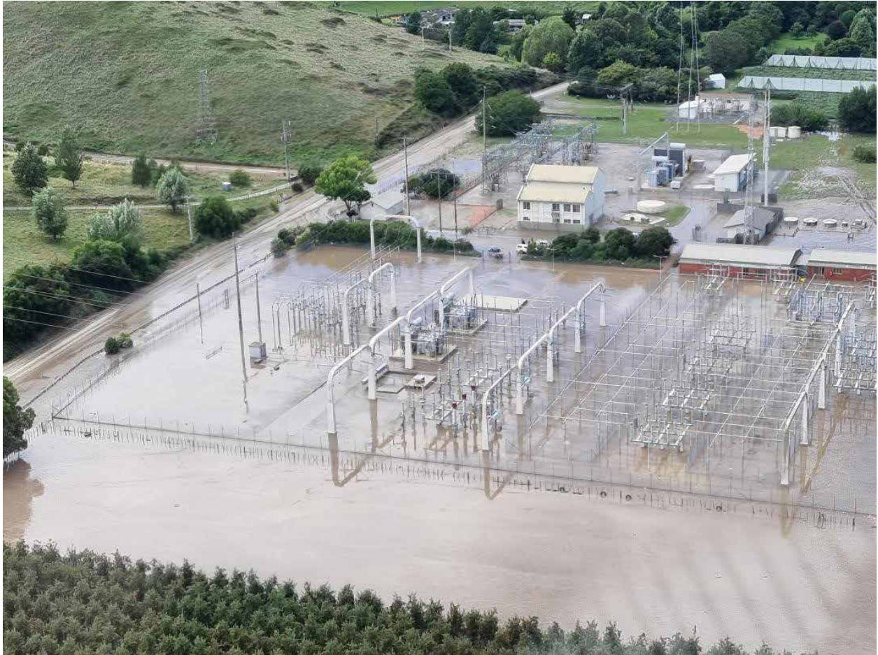
Figure 2.9 Transpower Redclyffe Substation 34
