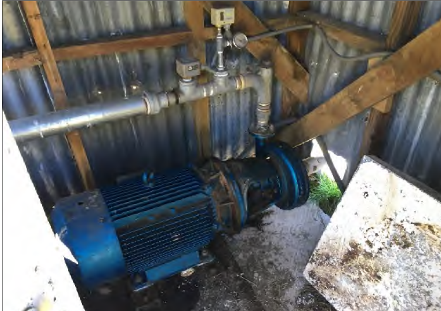
Figure 6. Well No. 2902 pump
