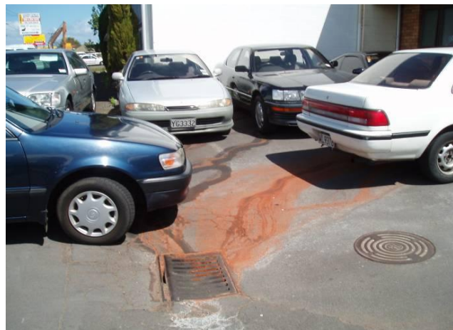
Example of Staining that Indicates Discharge of Contaminants into the Stormwater System
