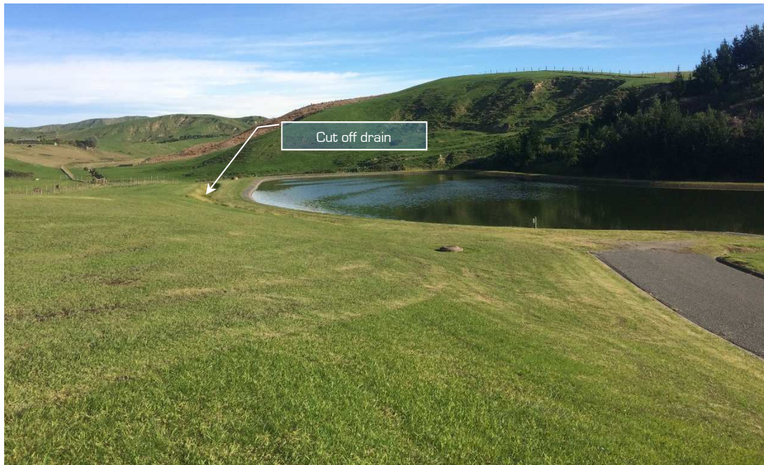
Figure 7: Western limit of secondary treatment pond. Note cutoff drain and northern slope.
