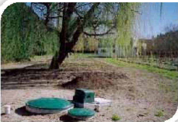
Parts of a secondary on-site wastewater treatment system that can be seen above ground.
