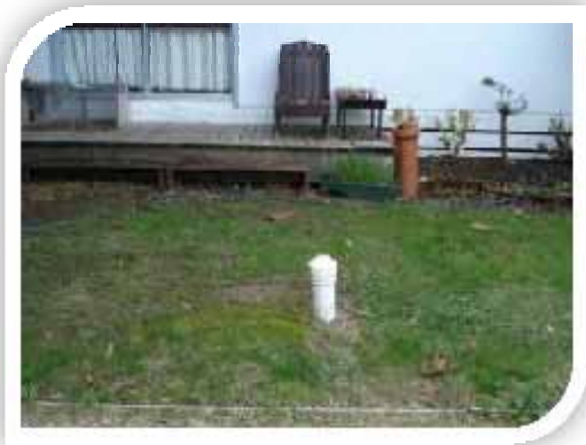
The air vent for the discharge field of an on-site wastewater treatment system
