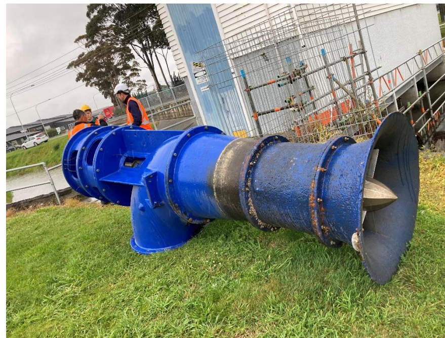
Figure 3: Plantation pump station and flood pump maintenance 2020
