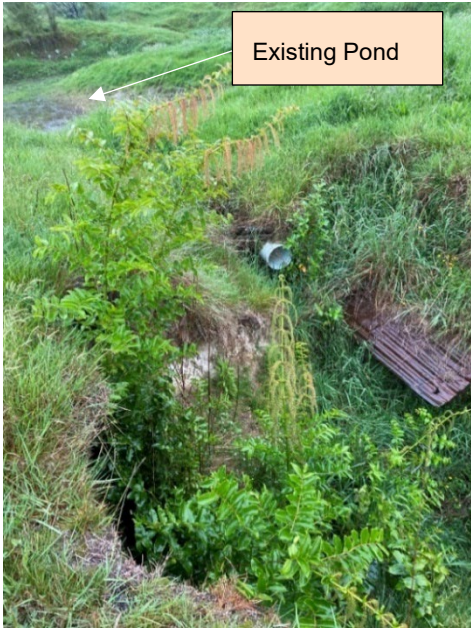
Figure 3-15 Piped drainage outlet for the existing pond. The pond can be seen in the background
