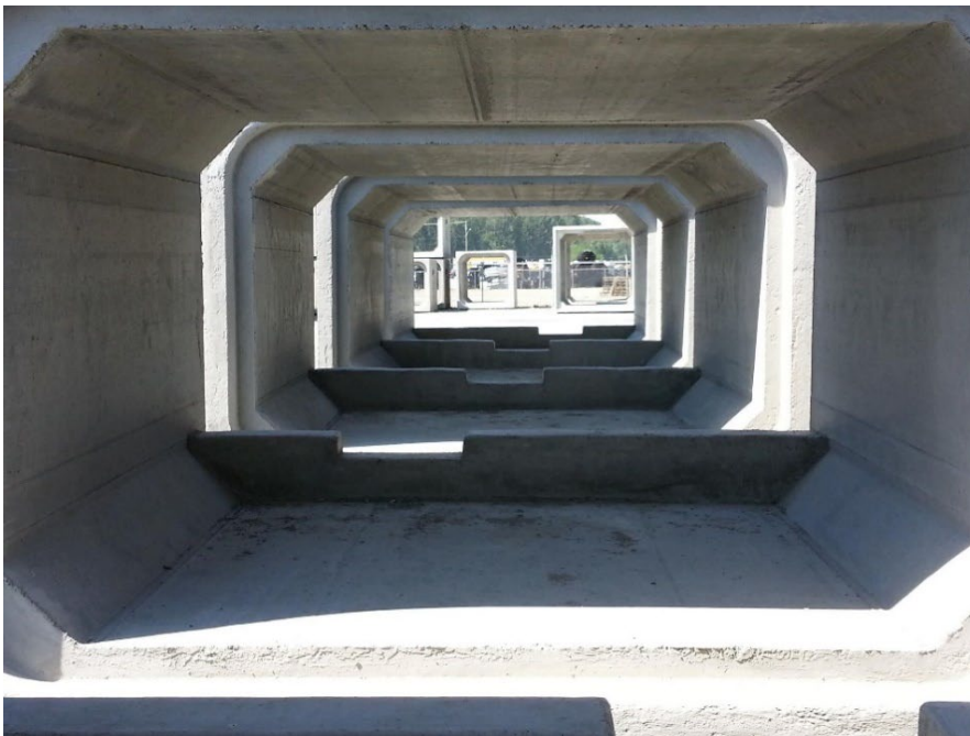
Figure 3-21 Concrete pre-cast baffles in box culverts for fish passage
